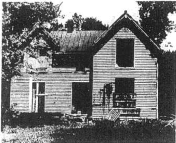
LATE STAGE: To be destroyed soon is this two-story frame building which once was the rectory of the St. Matthews Episcopal Church. The house is located at Westport Road and St. Matthews Avenue.
